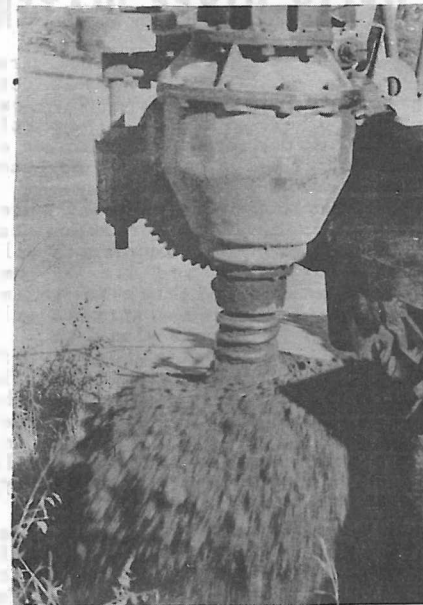
WHIRLING SCREW BRINGS OUT EARTH. DUMPS IT BESIDE BIG HOLE FOR LIGHT POLE ON TAVERN ROAD. THIS IS GREAT TIME SAVER.
